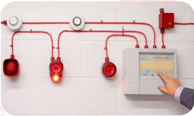
Fire Alarm System
