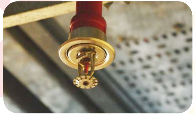
Fire Sprinkler System
