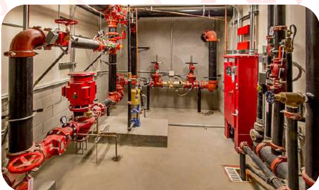
Fire Pumps + Panel
